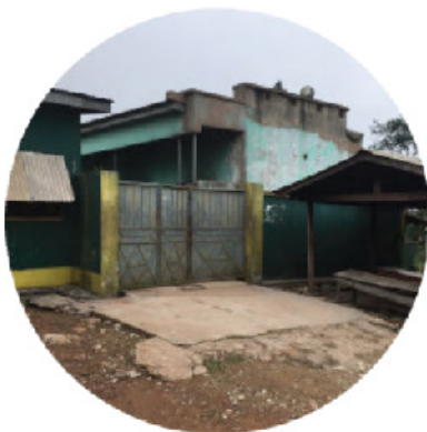
A dilapidated kitchen and pantry at Nifa Senior High School
