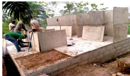
Workers erect walls for NAA's 10-seater biofil toilet system for Nifa Senior High School
