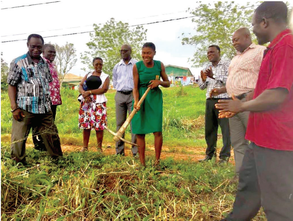
NAA President Nick Opoku joins the school community to turn the first sod for construction of the new toilet to start.
